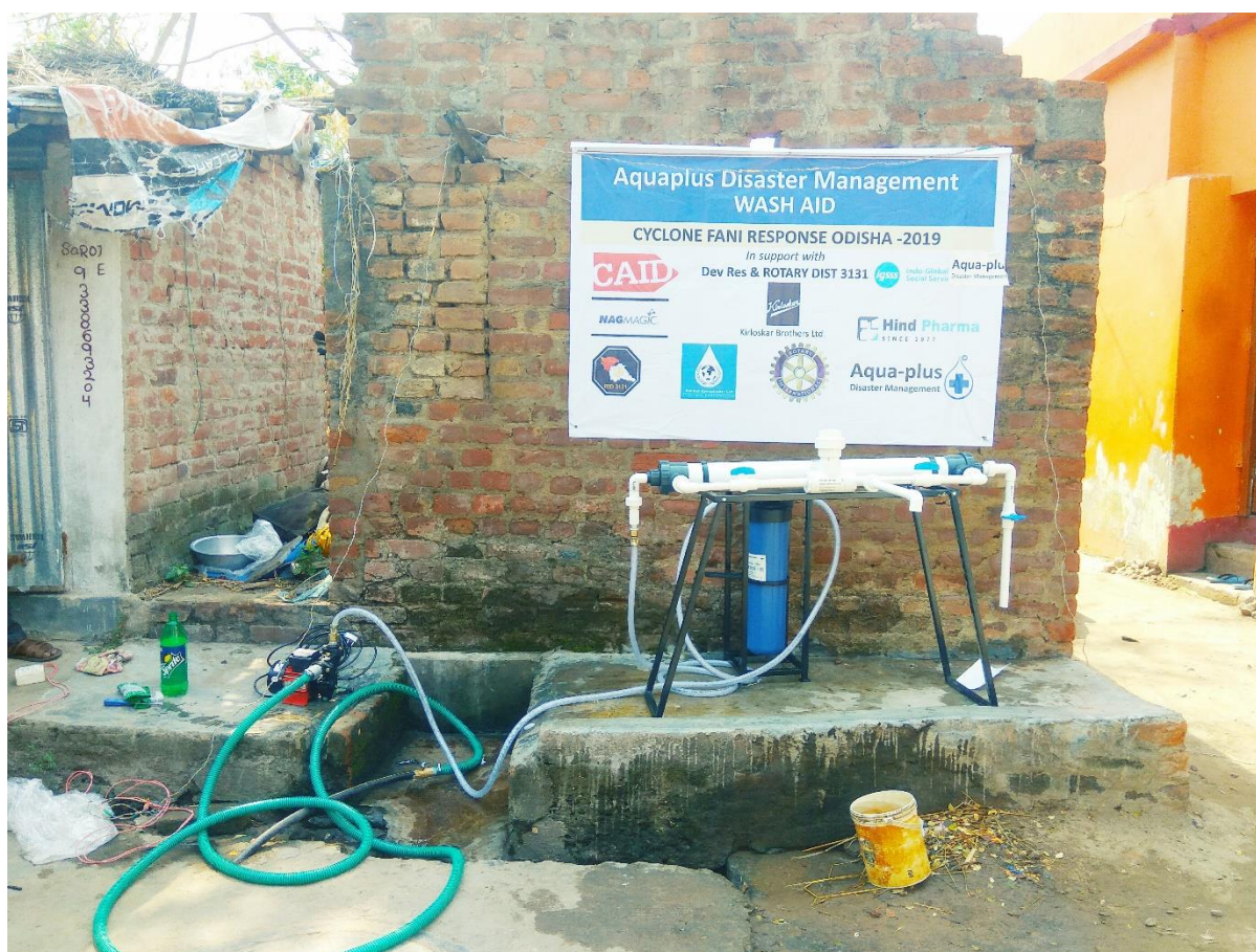
Installed the AP 700 Water Treatment Plant with Kirloskar pump
