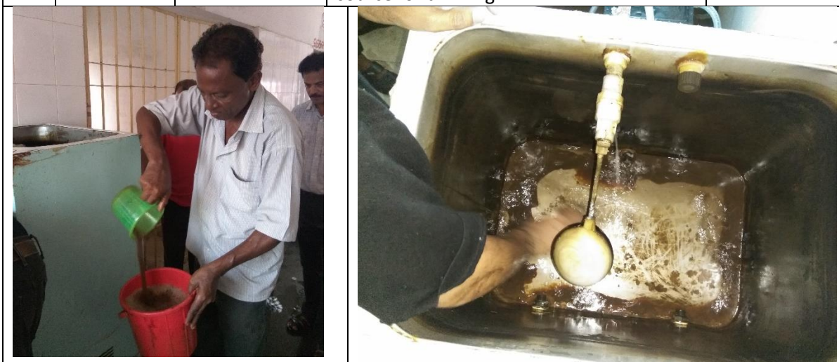
Team cleaning the tank before connecting to the AP 700 water treatment plant
