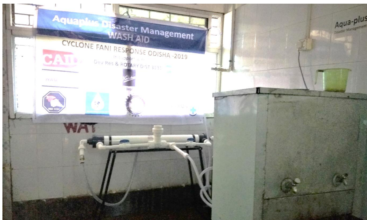
AP 700 Water Treatment Plant installed along water cooler
